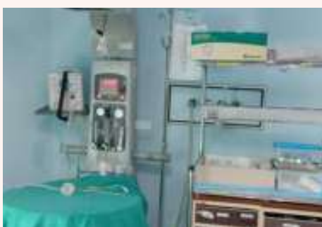
Radiant warmer in OT with emergency trolley
